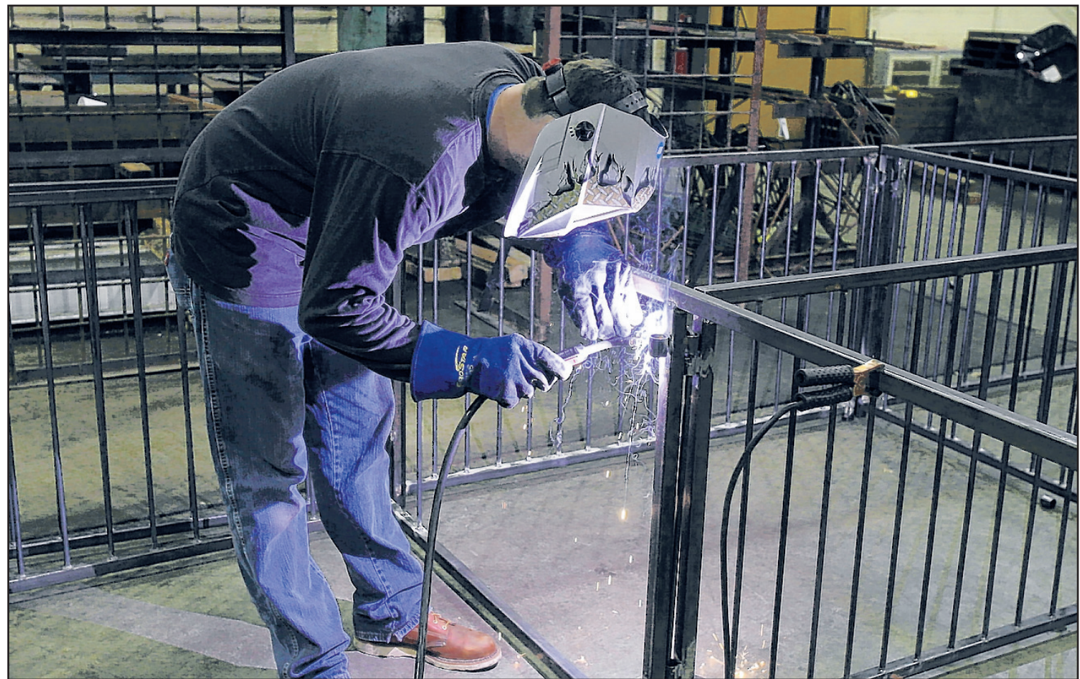
Tribune Photos/GENE KAISER Brett Fairchild, a local ironworker apprentice, welds a side of one of the 96 swine pens the South Bend Ironworkers Local 292 are constructing for the Berrien County Youth Fair set for Aug. 16-21.
